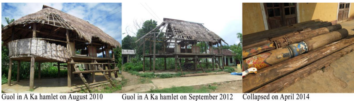
Figure 2: Deterioration process of Guol house in A Ka hamlet
