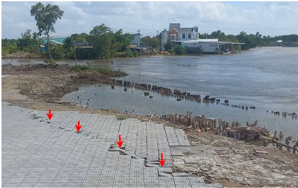
Figure 1. Riverbank erosion in Nguyen Van Thoi commune, Ca Mau province. (Photo: N.X.Nam, 2025)
