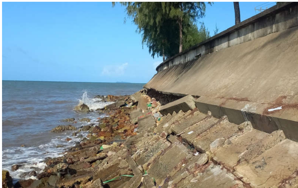
Figure 2. Erosion destroys concrete seawall along the coast of Kien Luong, An Giang. (Photo: N.X.Nam, 2025)
